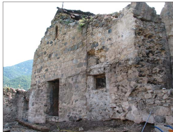
The chapel adjoining the western part of the southern facade of the church
