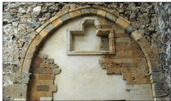
ANAMUR. A general view of the castle and its entrance tympanum after its "restoration"
