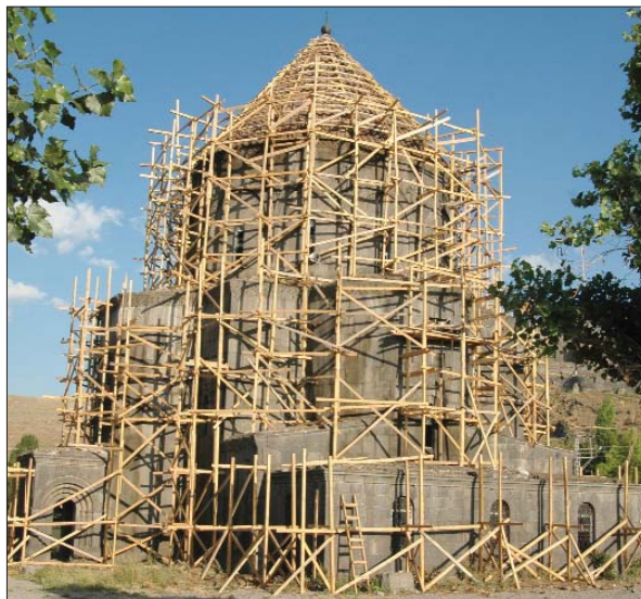
KARS. Arakelots Church before and during its “restoration”
